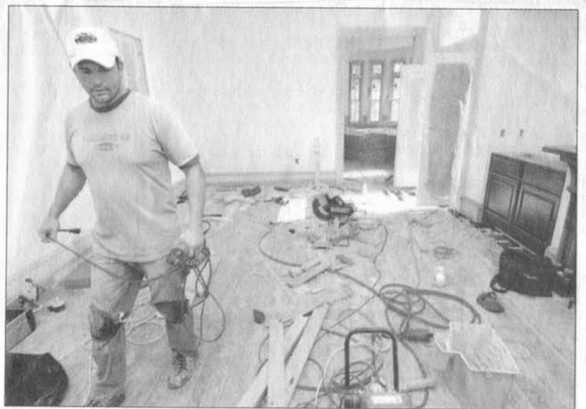
John Giddings of ABC Flooring makes complex and timely repairs to the wood floors of the home’s master bedroom Thursday afternoon.
